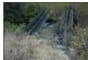
A burnt out bridge
